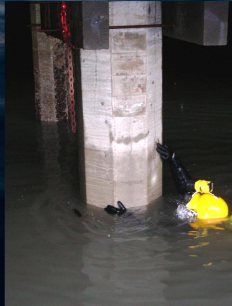
DEF in Concrete Piles
