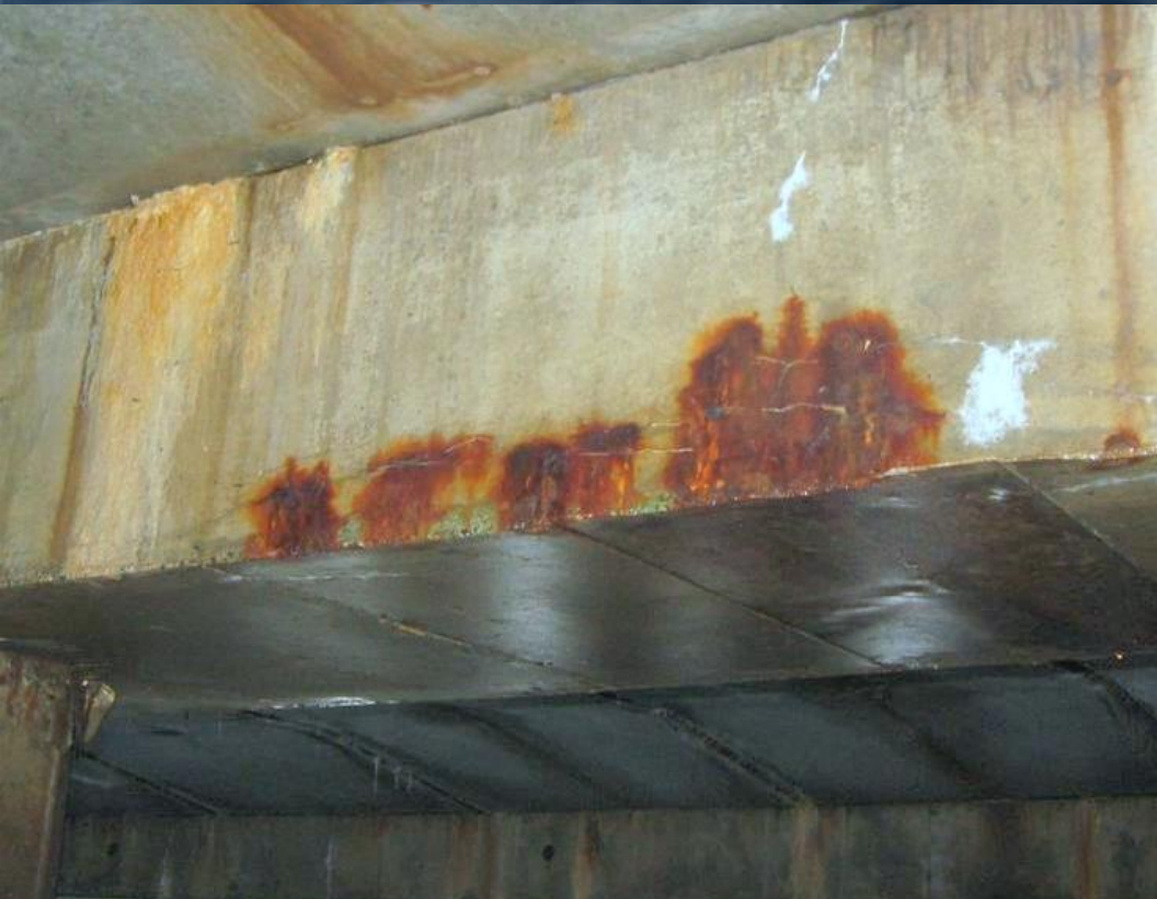
Concrete Pile Cap Distress
